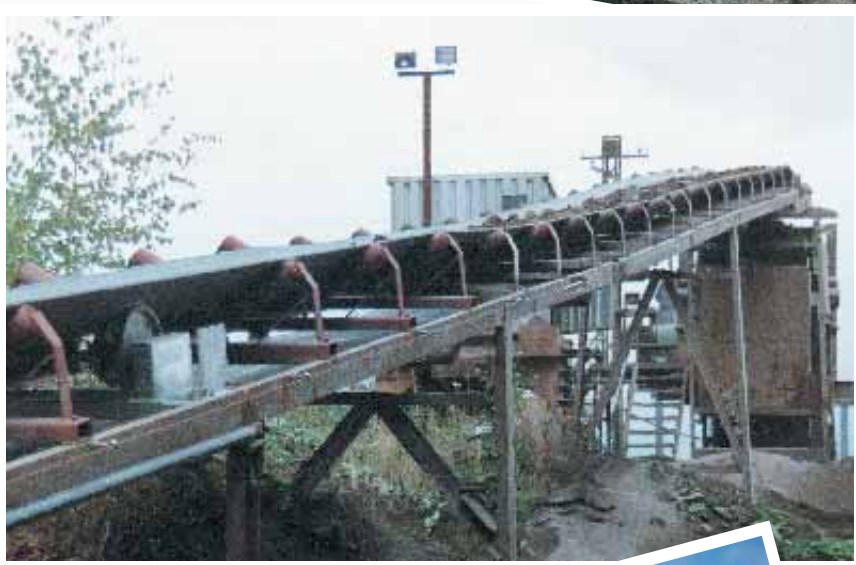
Example 4: FMS belt weigher in discharging conveyor of a stationary crusher. Capacity 400 t/h.
